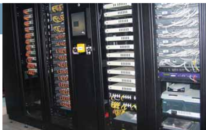
One of the Environmental Racks installed within all of the Department of Labour's server rooms throughout the country.
